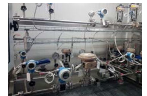
Realiz. Piping skid in container
